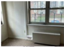
Demonstrating Energy Saving Performance of Heat Pump Technology in New York State (FGAI)
