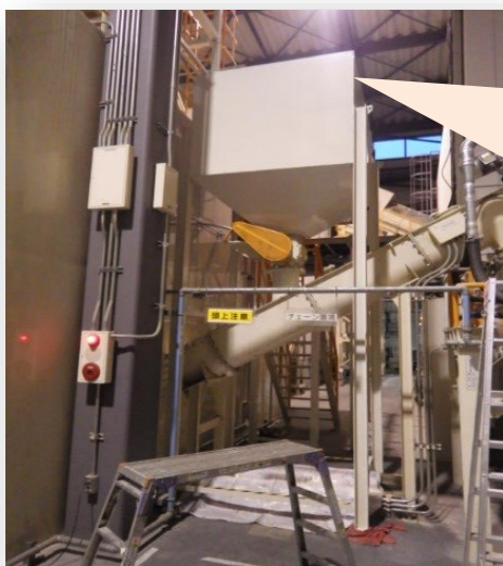
Dust collecting device introduced at Fuji Eco Cycle Co., Ltd.
