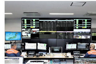
Fire and emergency communication command system
