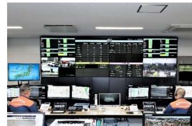
Fire and emergency communication command system
