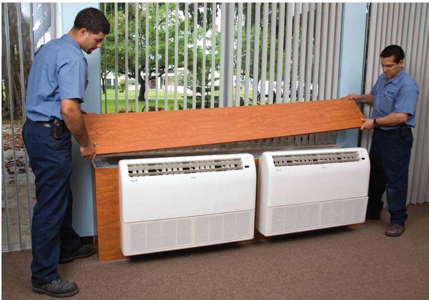
Installers Eugene Roman and Eli Castro put the finishing touches on an indoor-unit installation.
