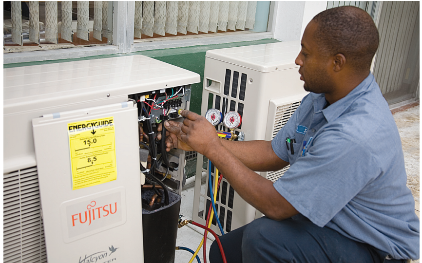
Startup service technician Garfield Thompson performs startup on one of the condensing units.
