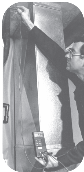
FIGURE 48 TEMPERATURE RISE MEASUREMENT
